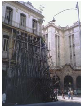
Repairs needed in Havana
